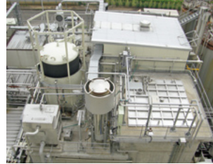
Anaerobic wastewater processing equipment at the Kisogawa Plant
