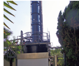
Biological desulfurization equipment
