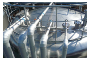
Storage tanks for recovered water
