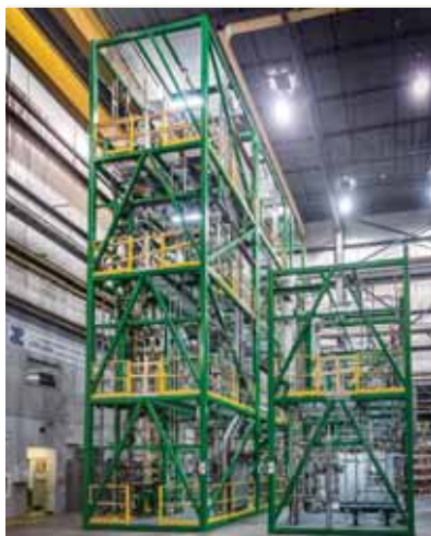
▲ A section of the testing plant of Anellotech, Inc.
