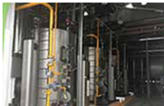
Newly installed boiler at the Beam Suntory Sauza Plant in Mexico
