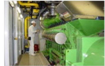
Cogeneration system at Tonegawa Brewery
