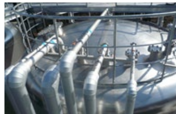
Reuse of water recycled at each stage of cleaning stored in 200 ton tanks
