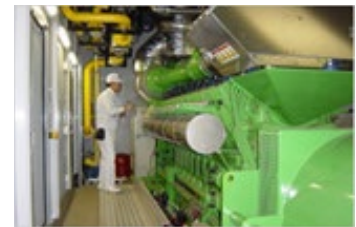
Cogeneration system at Tonegawa Brewery
