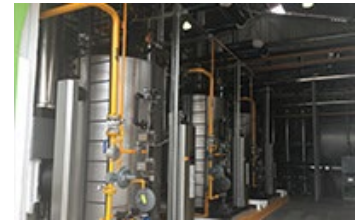
Newly installed once-through boilers at the Beam Suntory Sauza Plant in Mexico
