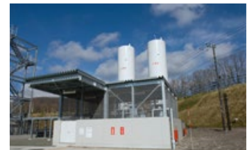
Liquefied natural gas facility at Okudaisen Bunanomori Water Plant of Suntory Products Ltd.
