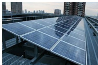
Solar power generation system of the Odaiba office
