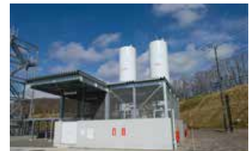
Liquefied natural gas facility at Okudaisen Bunanomori Water Plant of Suntory Products Ltd.
