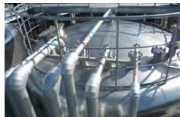
Reuse of water recycled at each stage of cleaning stored in 200 ton tanks
