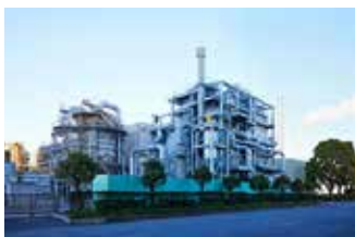
Biomass boiler (Chita Distillery)
